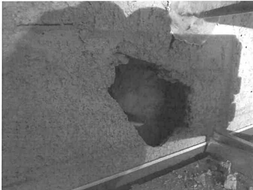
Buried pipe insulation behind block wall in 1 st Floor Women's Room – Old Extension.
