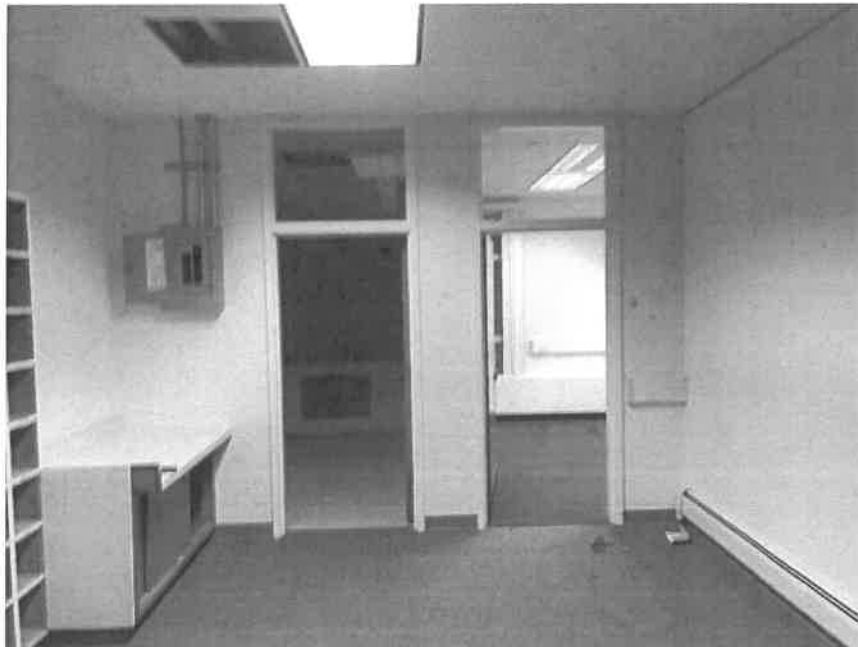
Administrative back offices. Note – mastic beneath carpet/floor tile in this area is ACM.
