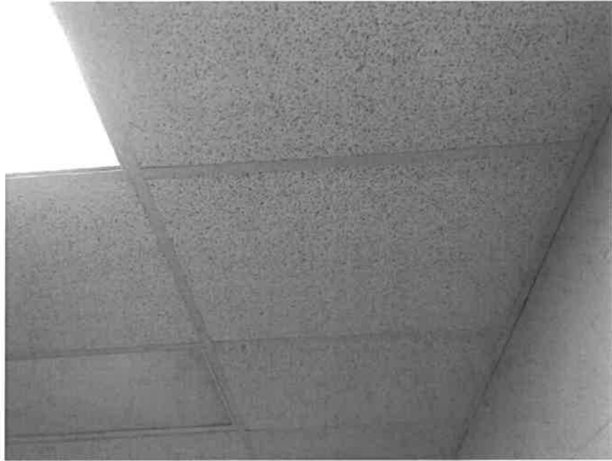
2' x 2' pindot ceiling tile
