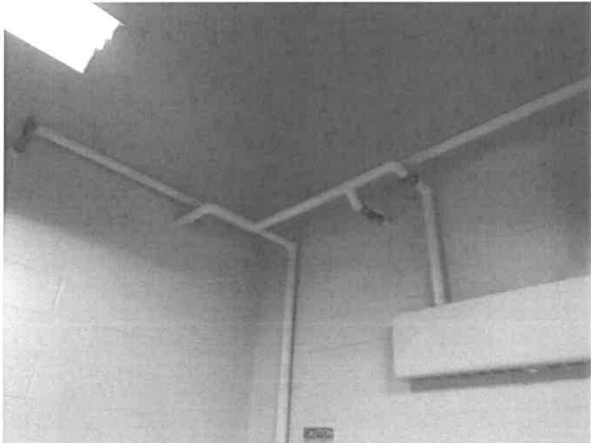
ACM pipe fittings in storage room off stage
