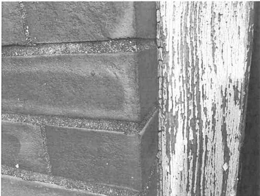
ACM exterior door caulk on Main Building and Old Extension doors
