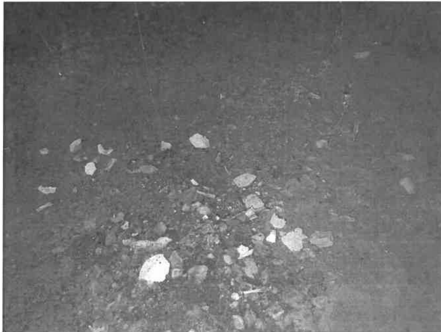
ACM pipe fitting debris in Kitchen Crawspace
