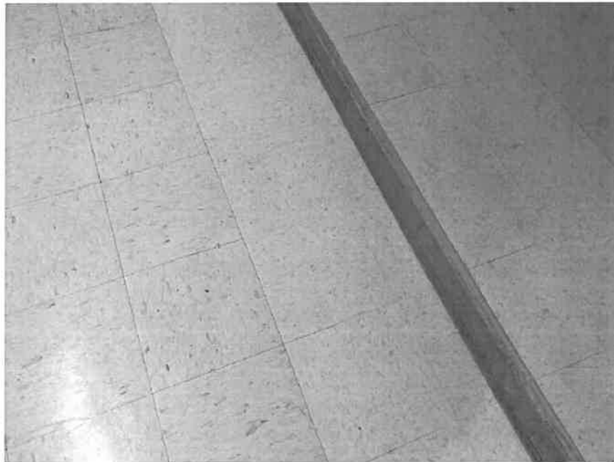
12" x 12" light pink floor tile and 12" x 12" light grey streaked floor tile in New Extension.
