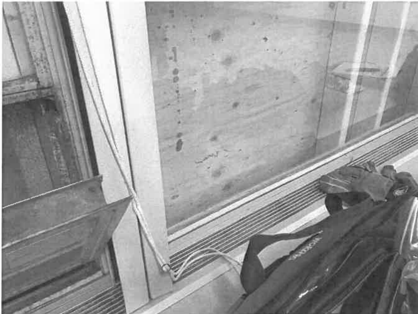
Typical classroom windows in Old Extension. Windows here have ACM window caulking and glazing.
