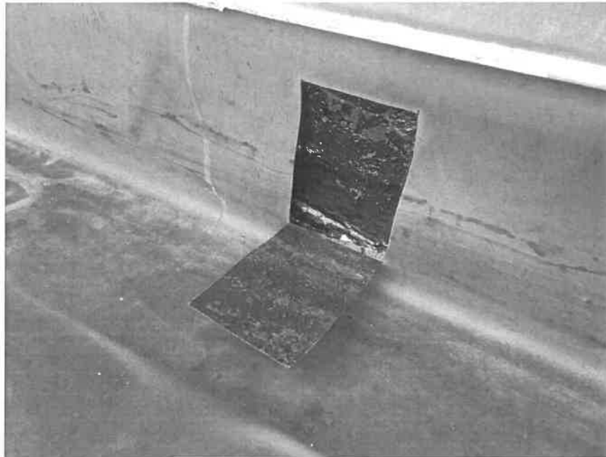
ACM black mastic on parapet roof – Crossover Roof
